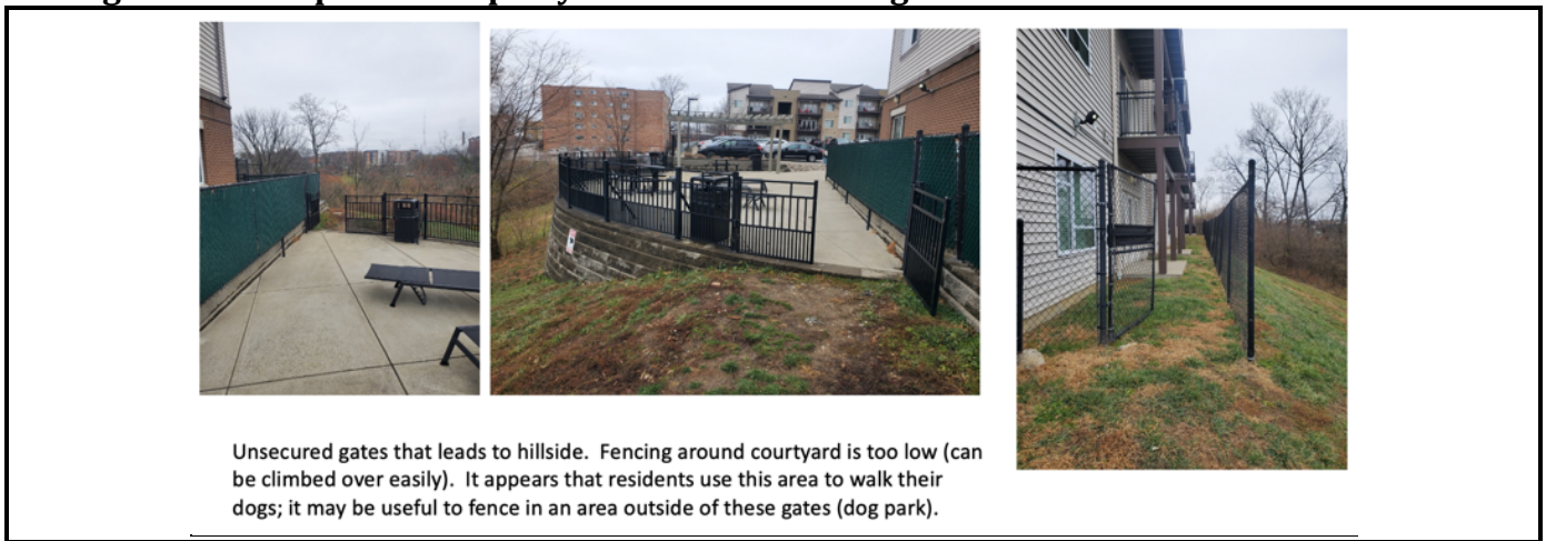
Figure 6: Examples of Property Assessment Findings at 2420 Ohio
