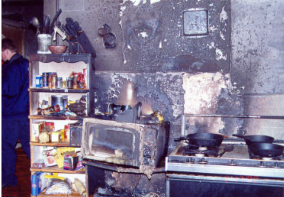
This house was damaged by a meth lab explosion.
