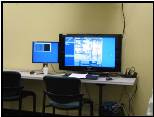
FIGURE 1. Picture of remote viewing station at initial installation
